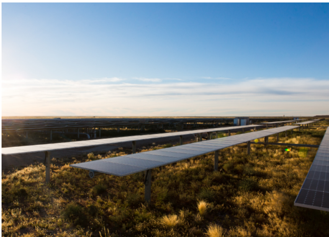
The 75 MW Mulilo Sonnedix Prieska solar project
